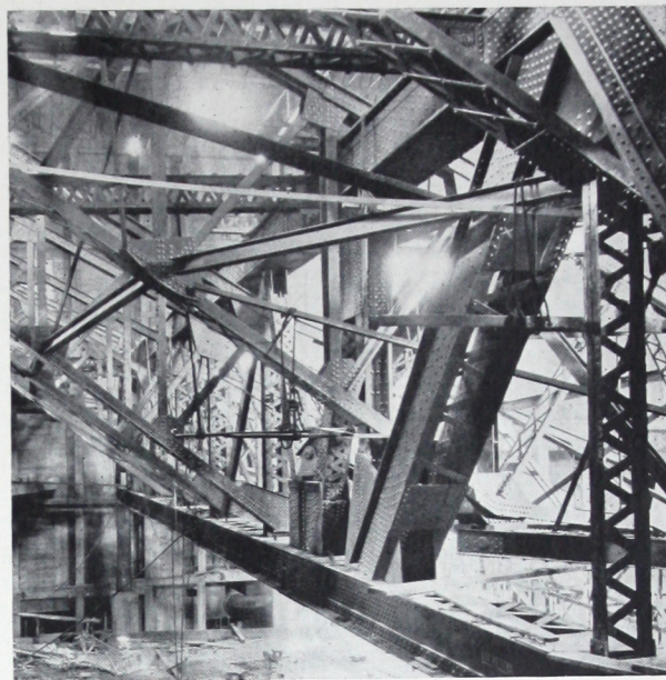
MAIN BALCONY TRUSS SHOWING INTRICACY OF CONNECTION DETAILS AND PIN CONNECTION OF JACK TRUSS TO STEEL CASTING ON MAIN TRUSS. ELECTRIC WELDING WAS USED TO OBTAIN METAL-TO-METAL CONTACT WHERE INCLINED SURFACES MADE IT DIFFICULT TO MILL ACCURATELY
